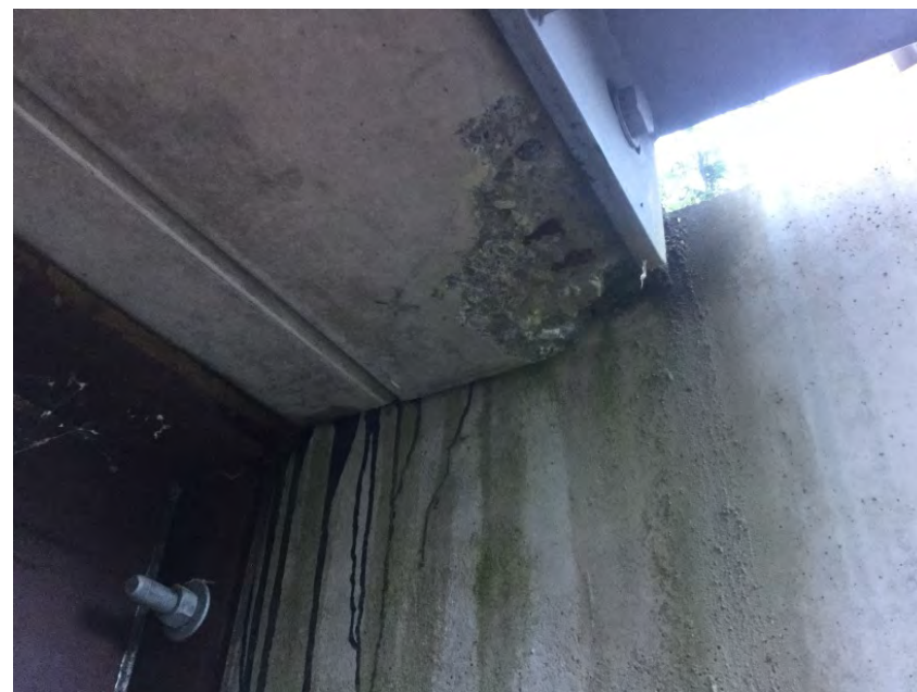
Damage under panel 1 at downstream left bank
